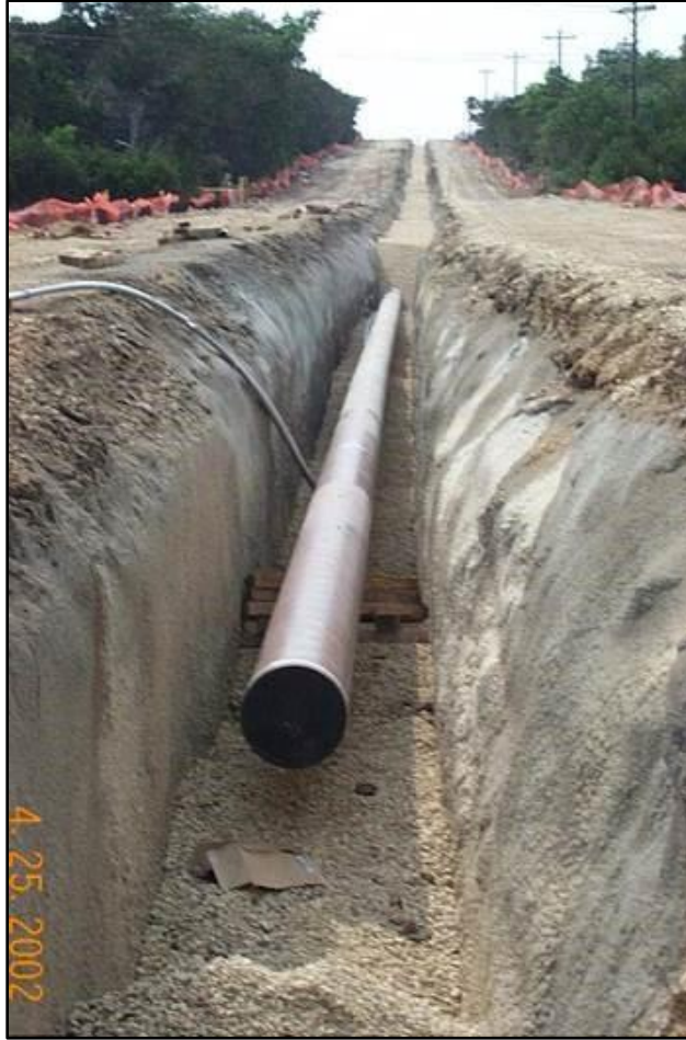
Figure 9. Longhorn Pipeline with gunite lining of trench. Photo courtesy of Barton Springs/Edwards Aquifer Conservation District.
