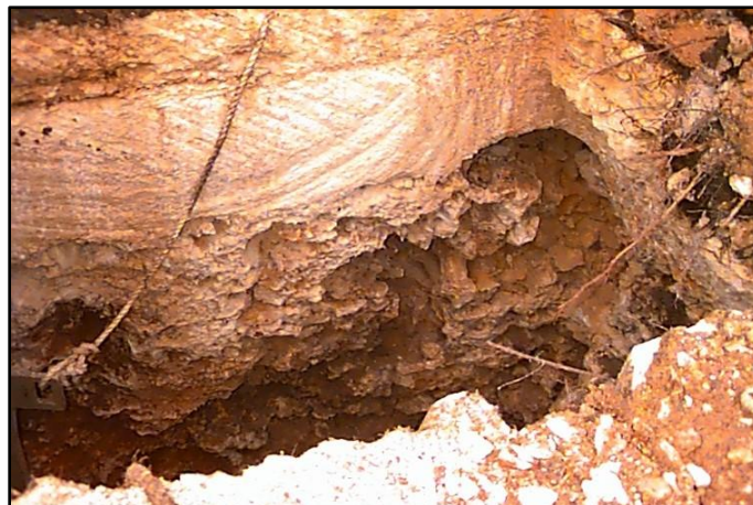
Figure 10. Karst voids in the trench of the Longhorn Pipeline. Photo courtesy of Barton Springs/Edwards Aquifer Conservation District.
